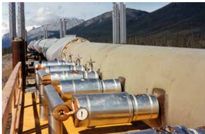
Multiple injection ports were required to achieve high Gel DRA dosage rates
