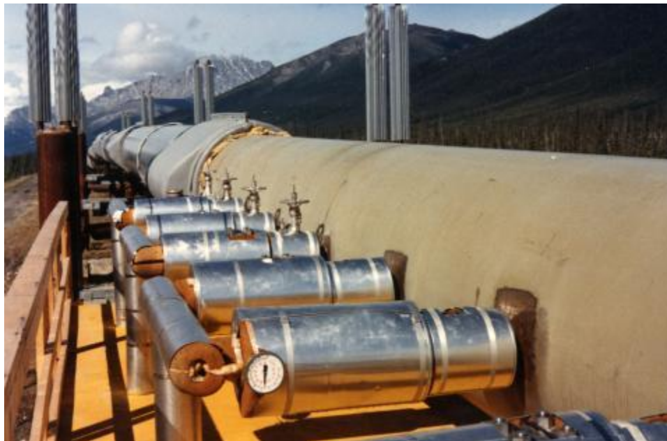
DRA injection site on crude oil pipeline; Source: LSPI
