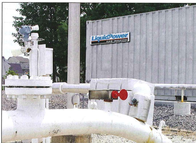
Injection skid installed at pump station to accommodate increased flow improver levels.
