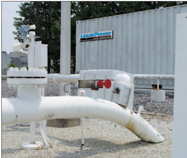
The LiquidPower™ Flow Improver injection skid injects RP™ II Flow Improver into ConocoPhillips' East Line at the Chelsea Terminal in Trainer, PA.
