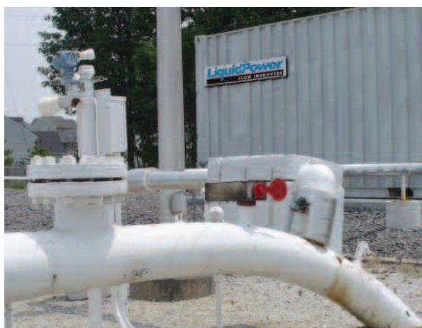
The East Line, an 8-inch diameter pipeline, delivers refined products to the New York City market.
