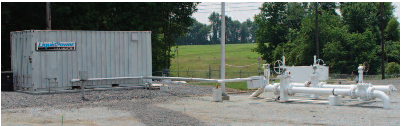
The CSPI injection equipment injects RP II™ Flow Improver into the ConocoPhillips East Line at the Chelsea terminal in Trainer, Pa.
